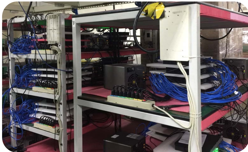
Test for all RJ45 ports
